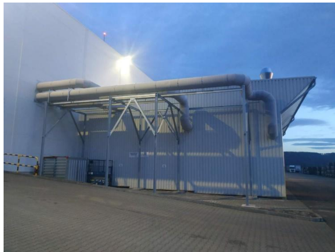
Air-conditioning systems - piping
