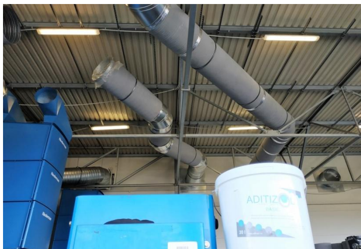
Air-conditioning systems - piping
